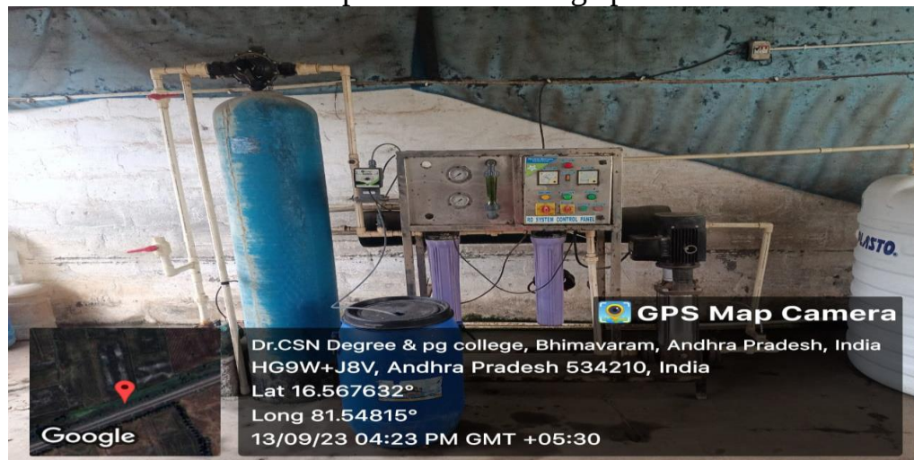
RO water plant in our college premises
