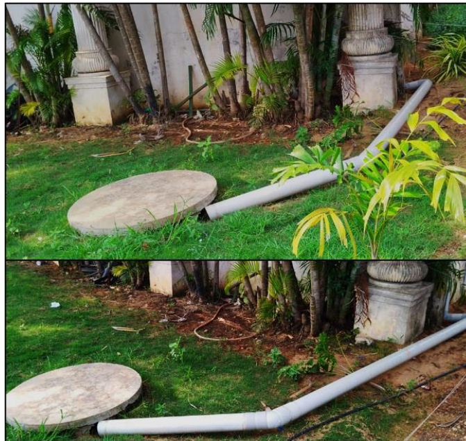
Rainwater harvesting implemented and maintained properly for water conservation
