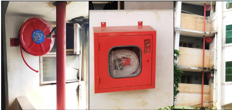
Fire Hydrant System implemented in the buildings.
