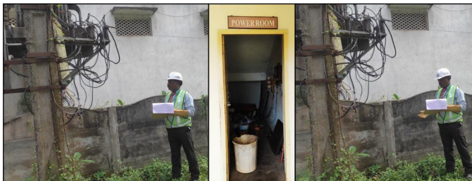
Energy conservation facilities observed in the Campus
